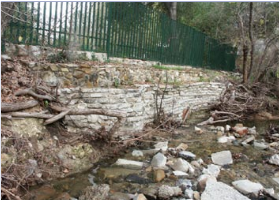
Before Restoration: Streambank was vertical and armored with stacked concrete and asphalt rubble.
